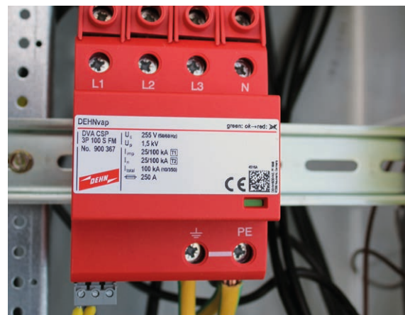
Figure 4 Protection for the AC power supply unit of a base station with DEHNvap CSP 3P 100 S FM
